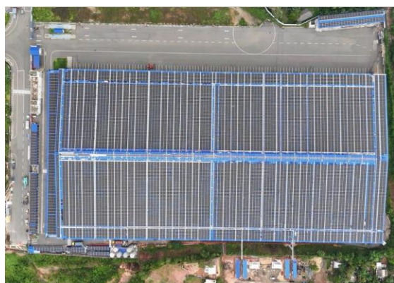
Figure 2: Aerial site view of rooftop installation (EGFI, 2023)
