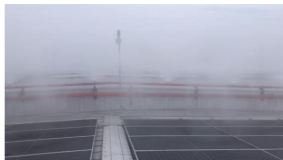
Figure 4: Operational test - Open Sprinkler Line in Action
